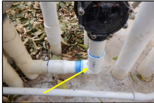
Pipes exposed to direct sunlight
