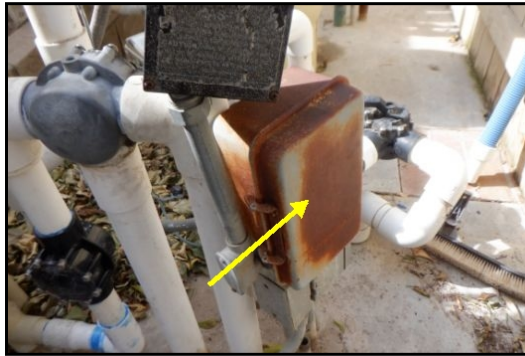
Rusted electrical box
