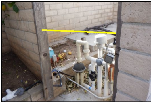
Enclosure unsafe condition
