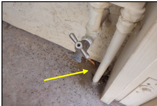
Leaking valve noted
