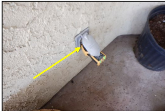
Not GFCI protected outlet
