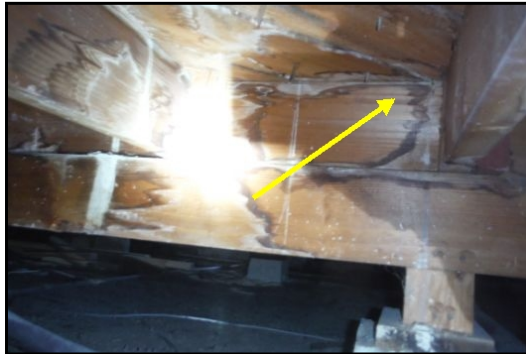
Evidence of dry past water damage
