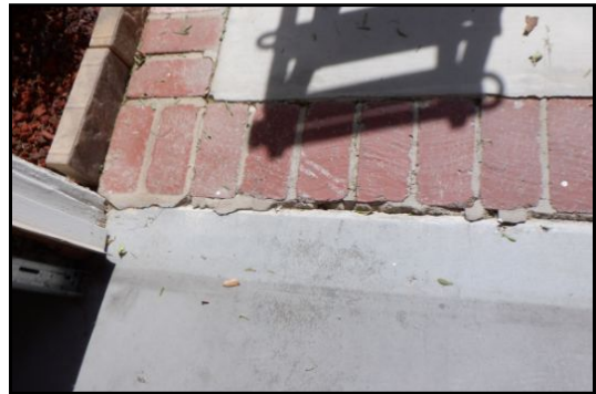
Garage floor lower at driveway
