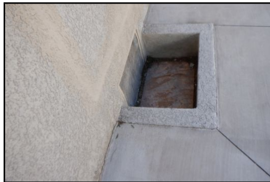
No concrete curb
