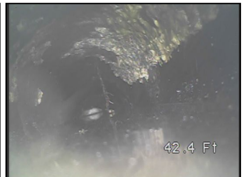
Possible bellies or settling pipe
