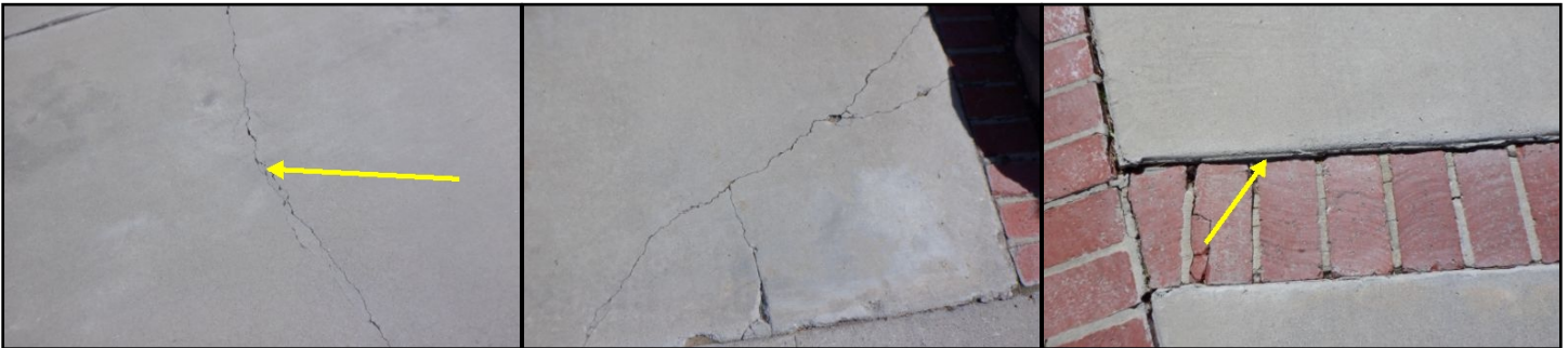
Cracks on driveway
