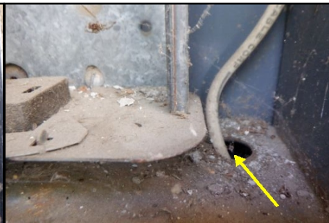
No bushing installed
