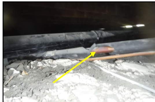
Missing/deteriorated refrigerant line insulation
