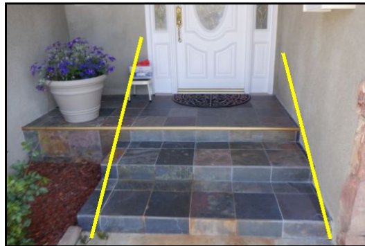
No handrail more than 2 risers
