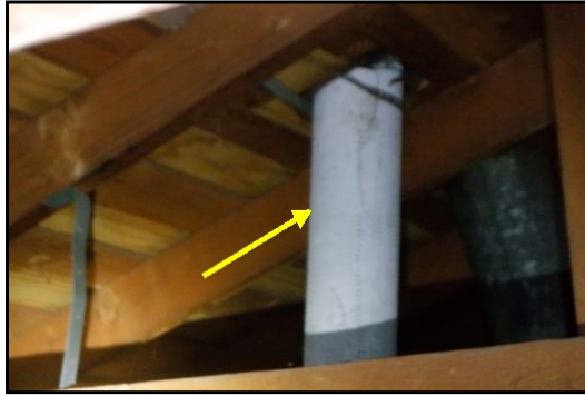
Possible asbestos materials
