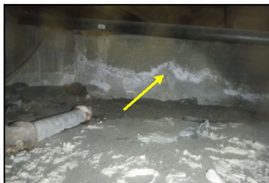
Efflorescence on foundation wall
