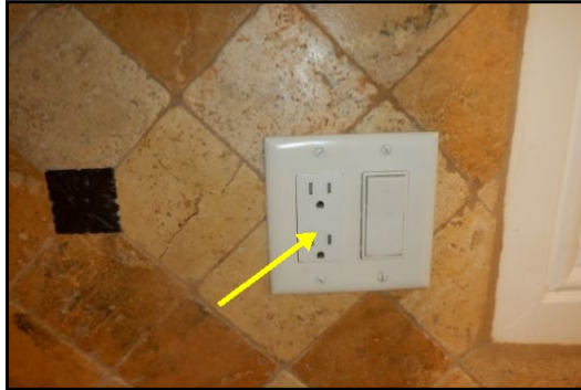
Not GFCI protected
