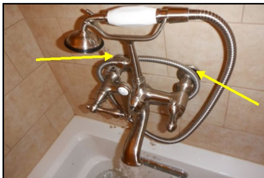
Loose faucet from wall
