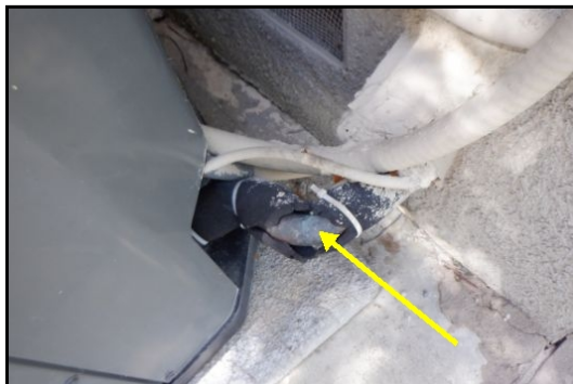
Missing/deteriorated refrigerant line insulation
