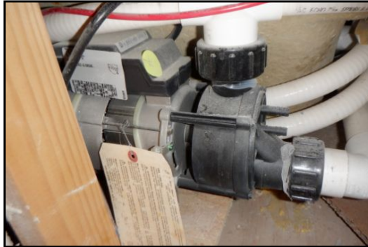
GFCI protection was inoperable
