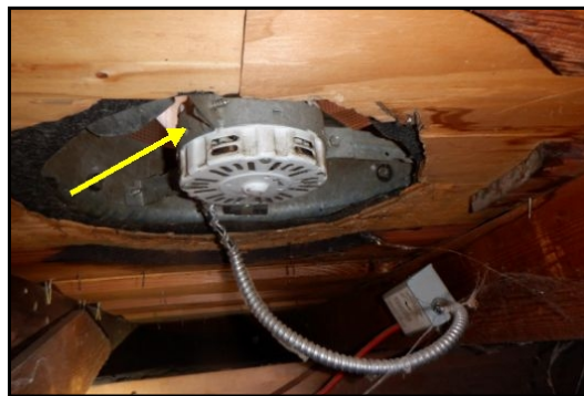
Inoperable fan noted
